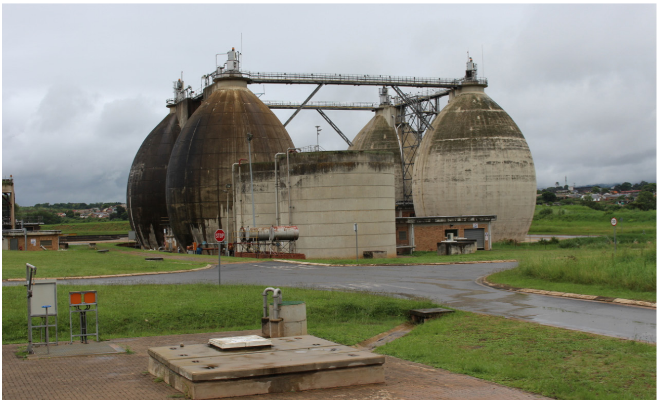
The anaerobic digesters, the Darvill works' most visually striking feature. Inside the heated eggs, bacteria break down organic waste in the absence of oxygen.
