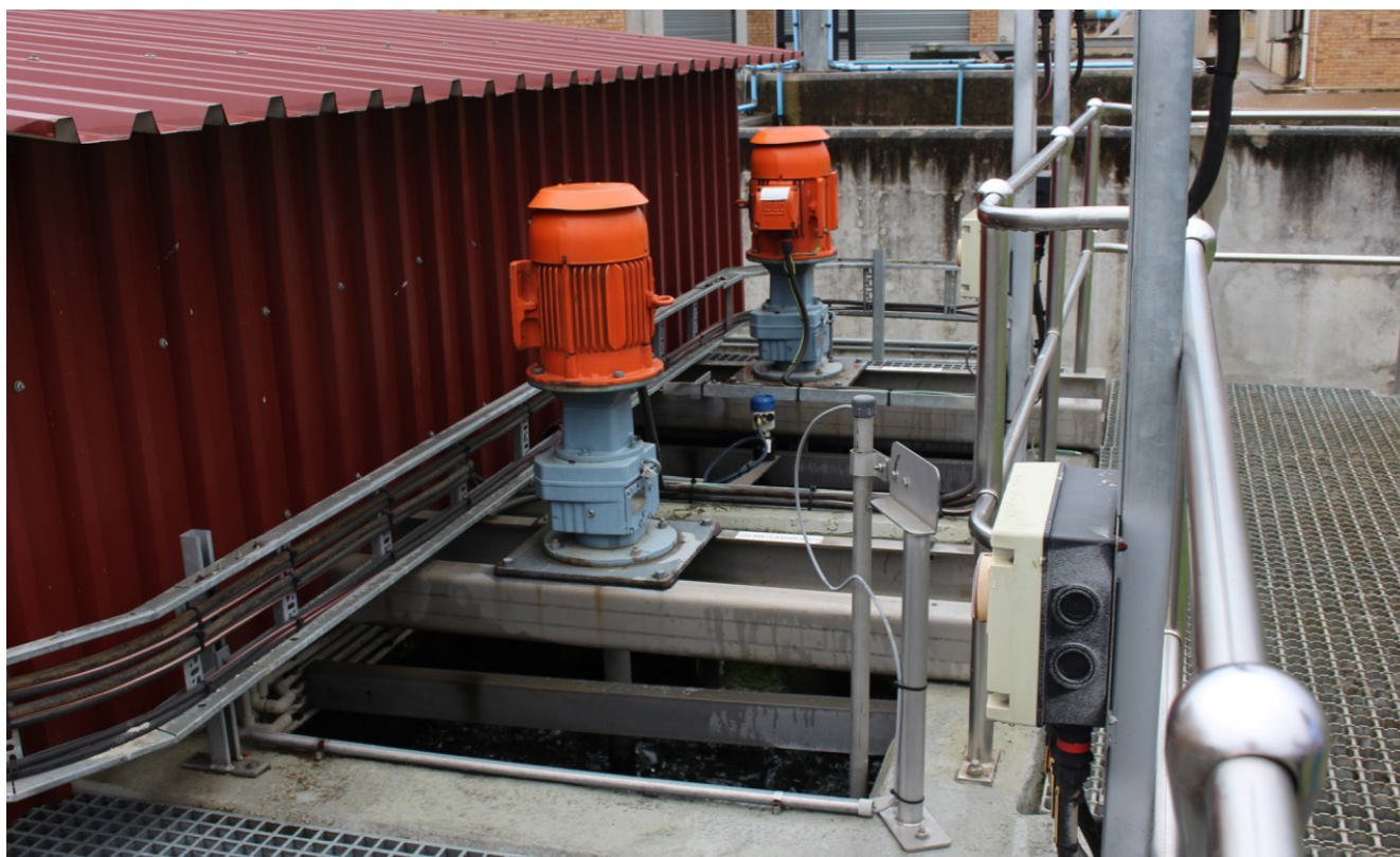
Flash mixing in the high-pressure wash plant disperses coagulants – aluminium sulphate and a polymeric coagulant – in the feed water. This helps suspended particles to clump together.
