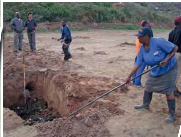
The sludge being buried. The project has created quite a number of jobs for the surrounding community.
