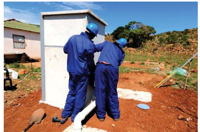
Community members were trained in the installation and maintenance of the toilet structures.
