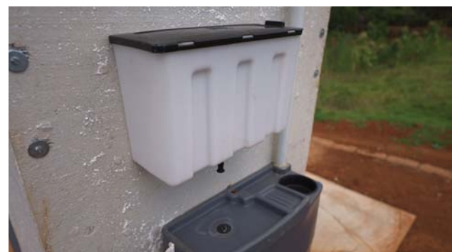
The toilets have also been equipped with handwashing stations.
