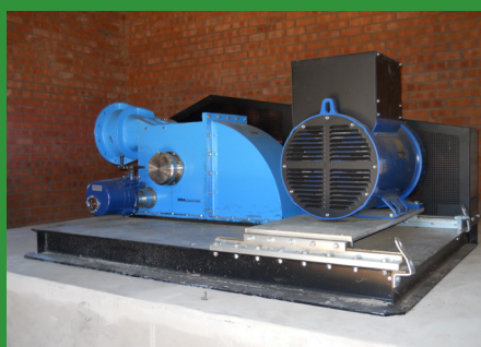
The conduit hydropower installation at Bloem Water.
