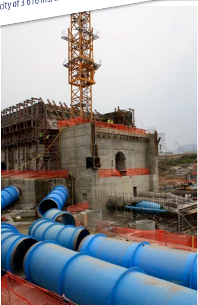
The enormous 2 m-diameter stainless steel outlet pipes. All the pipes are being manufactured at the DWA Central Construction workshops in Jan Kempdorp.
