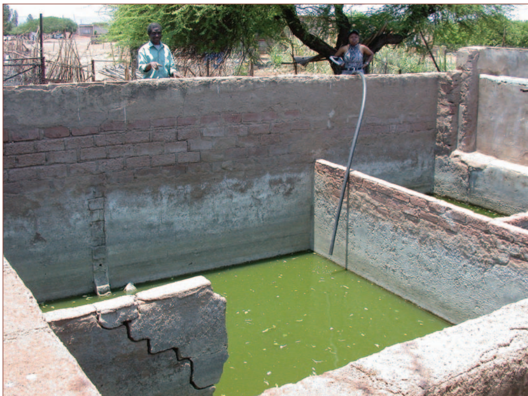
There are an estimated R100-million worth of facilities and hatcheries in the country. Most are dormant and some have fallen into disrepair.
