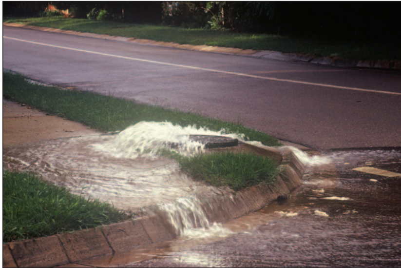
Extraneous flow can reduce the originally designed capacity of a sewage collection system.
