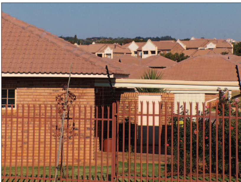
The illegal connection of gutter down pipes to sewer gullies and the paving of yards, especially in sectional title properties, are some of the leading causes of stormwater ingress.
