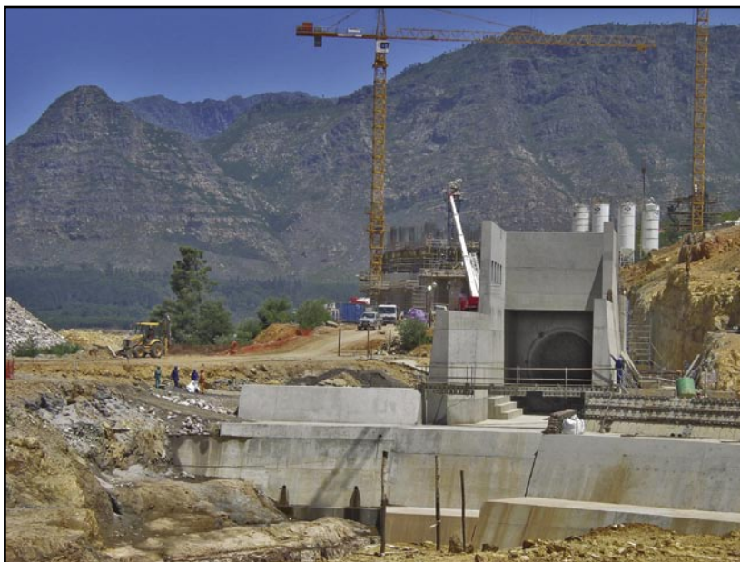
In November the Berg River was closed off by the dam, and diverted temporarily through the outlet conduit shown here.
