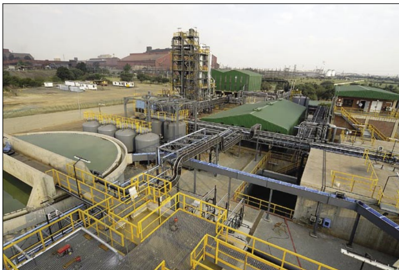
Mittal Steel South Africa's zero liquid discharge plant.
