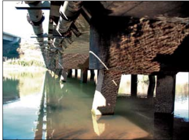
The piles of this bridge near the Mzimkulu River mouth have been exposed to a significant depth.
