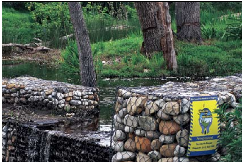
Higher in the catchment, restoration of the Prinskasteel River is being conducted as a Working for Wetlands project. Gabions have been built to arrest erosion that was resulting in loss of wetland habitat.
