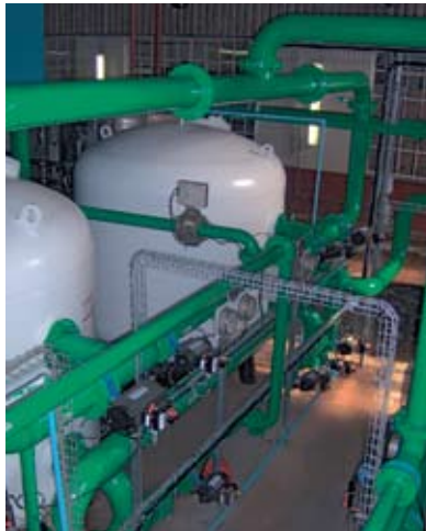
polishing filter. The chemical dosing and clarification units were reworked. Automated
