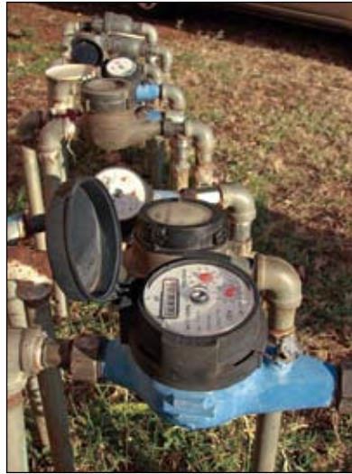
Non-compliant plumbing products can lead to unnecessary leakage and wastage of water.
