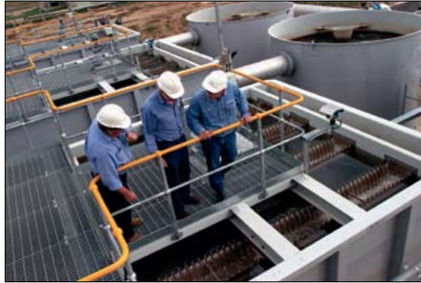
A water treatment plant employing the patented Actiflo clarification process.
