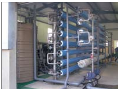
The recently commissioned Opuwo nanofiltration plant
