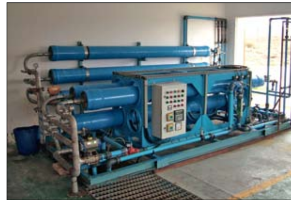
Research funded by the WRC led to the establishment of the first South African plant for drinking water purposes using membrane technology to be commissioned in 1990. The plant, situated at Bitterfontein, in the South Namaqualand, makes use of tubular reverse osmosis membranes.
