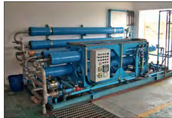
Research funded by the WRC led to the establishment of the first South African plant for drinking water purposes using membrane technology to be commissioned in 1990. The plant, situated at Bitterfontein, in the South Namaqualand, makes use of tubular reverse osmosis membranes.
