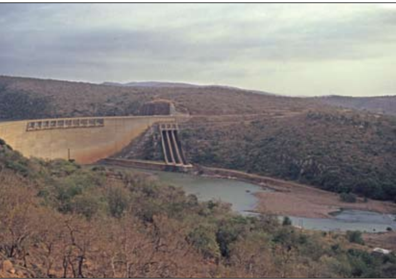
Pongolapoort Dam is a medium thin, double curvature arch dam with a gradual transition towards a gravity thrust block on the left flank.
