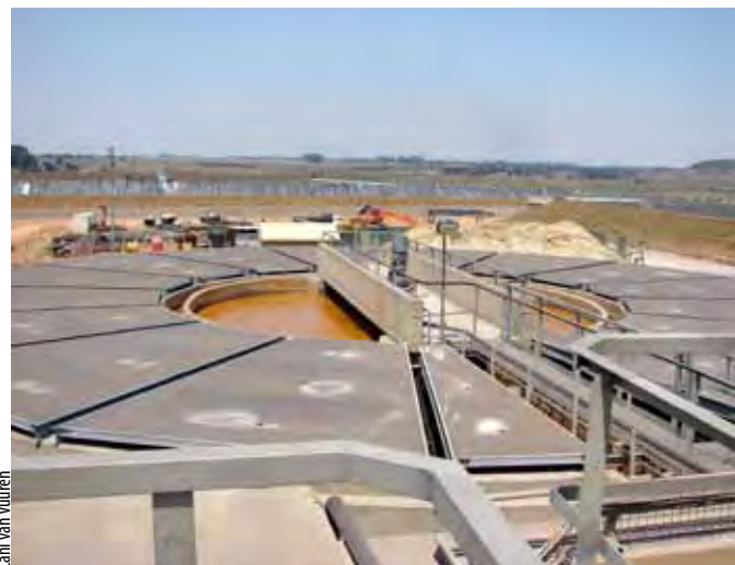
The Emalaheni Water Reclamation plant outside Witbank where polluted mine-water is treated to drinking water standard for the local municipality.
