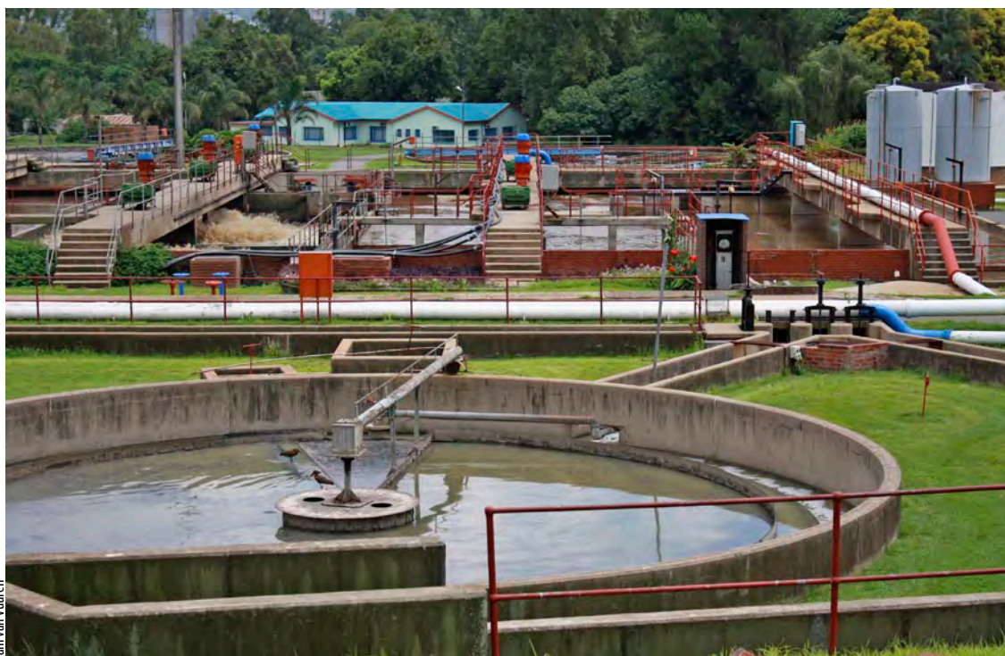
There remain big anomalies in the state of wastewater infrastructure between large metropolitan centres and rural areas.
