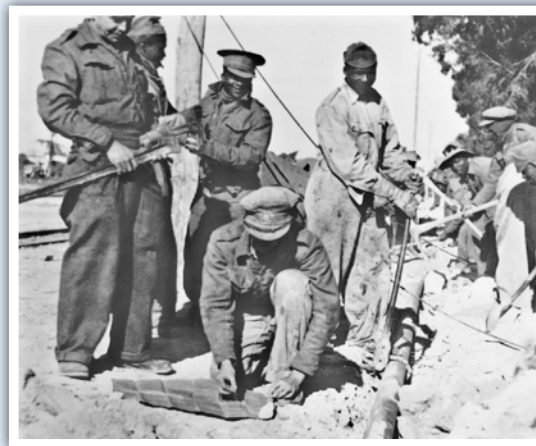
Above: Members of the 36th Water Supply Company, South African Engineer Corps, assisted by men from the South African Native Military Corps, lay a water pipeline at Benghazi, North Africa.
