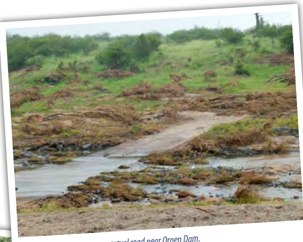
Damage to a causeway on a gravel road near Orpen Dam.
