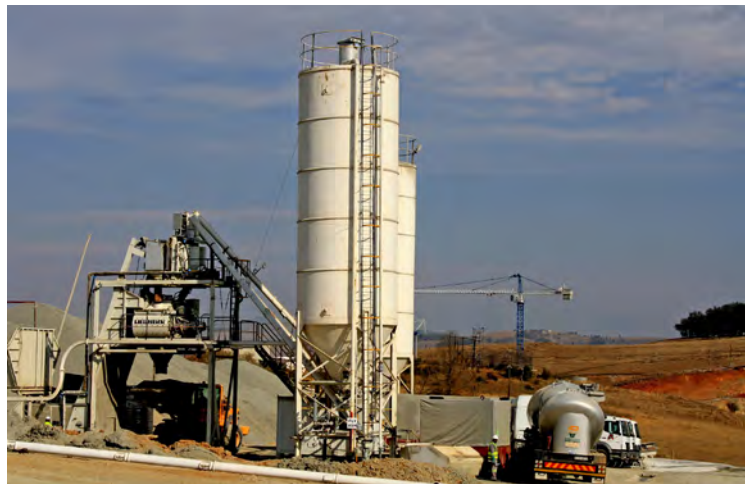
Top left: The Spring Grove batch plant. Around eight days' worth of material is stored on site.
