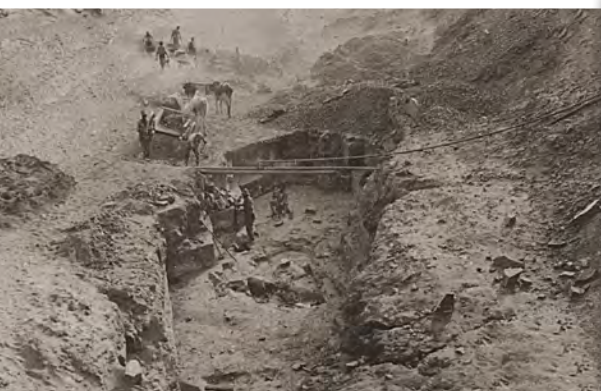
This photograph, taken in 1919, shows the excavation for the stilling and weir chambers of the Leeuw-Gamka Dam. The excavation was very irregular owing to cleavage found in the shale beds.
