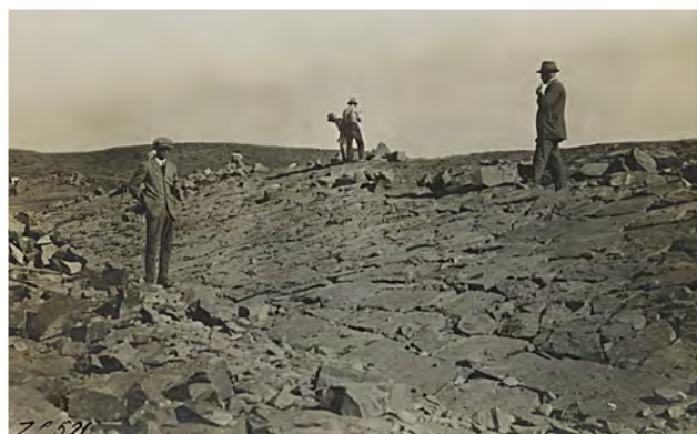
Construction of the stone pitching of the upstream slope of the Leeuw-Gamka Dam in 1918. Assistant Engineer E Jacklin is standing at the toe with Resident Engineer JJ Swalwell on the slope.
