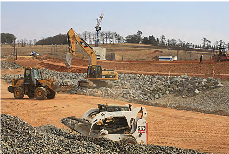
Rip-rap being placed against the slopes of the earthfill embankment. The embankment will be 11 m high and 315 m long upon completion.
