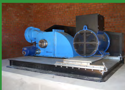
The conduit hydropower installation at Bloem Water.
