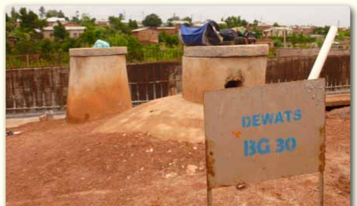
Construction of decentralised waste water treatment system at Kandundu project in Solwezi
