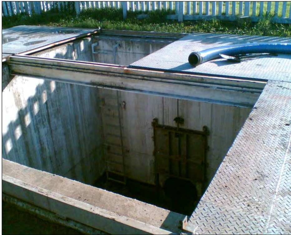
Figure 10.4: Sliding roof cover for silt trap (courtesy of BKS (Pty) Ltd)
