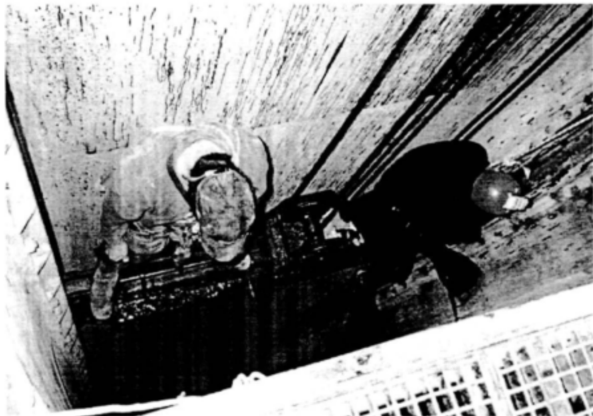
Figure 8.1.4-5 Lowering of the emergency gate at Roode Elsberg Tunnel
