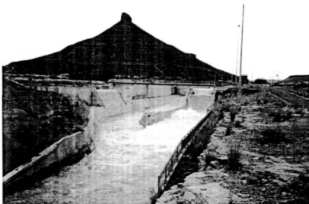
Figure 8.1.2-4 Orange Fish Tunnel flow measurement gauge
