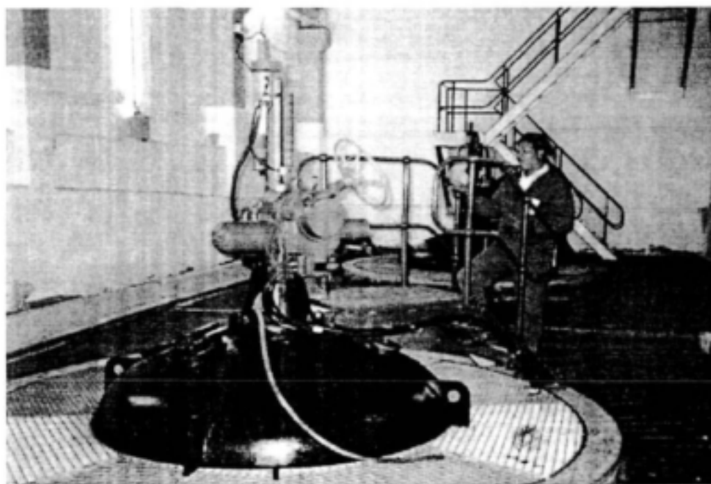
Figure 8.1.2-2 Orange-Fish Tunnel valve
