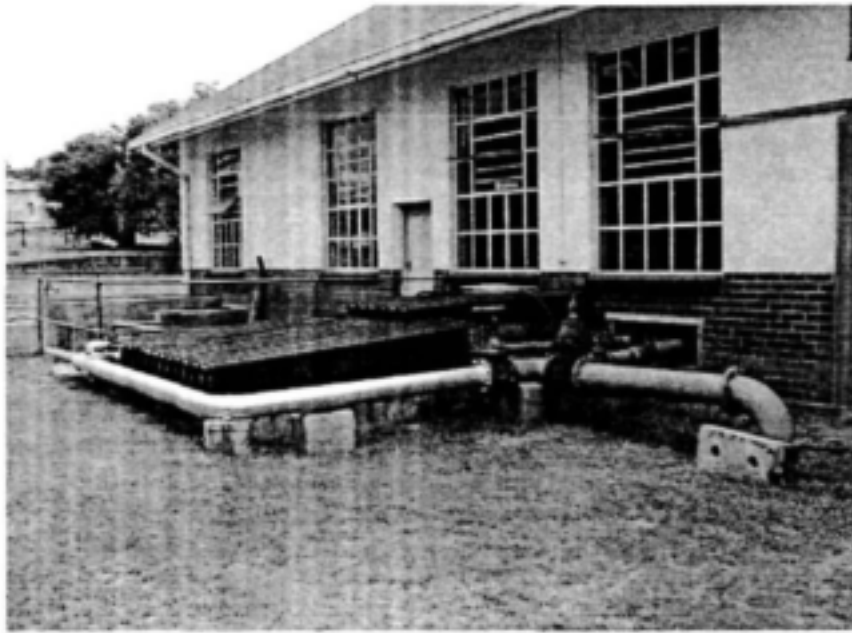
Figure 7.3.2-1: Pipe system at the hydraulic laboratory of the University of Pretoria
