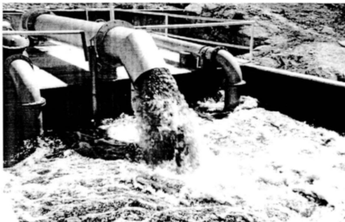
Figure 8.1.4-8 Bypass pipe at Roode Elsberg Tunnel
