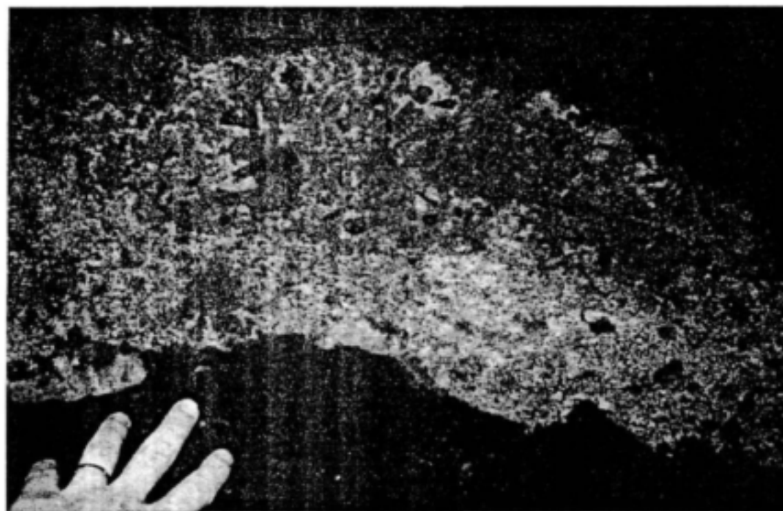
Figure 8.1.3-7 Exposed coarse aggregate after sediment removal due to emptying, Banghoek to Jonkershoek, Theewaterskloof Tunnel
