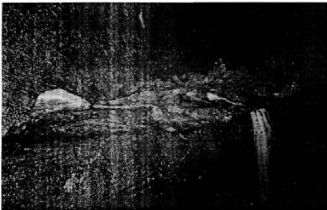
Figure 8.1.3-6 Deep scour in soft water corroded poor quality concrete, intake to Berg River, Theewaterskloof Tunnel
